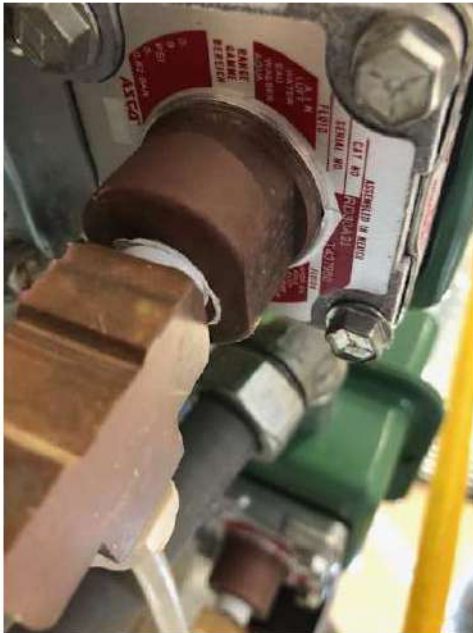
Part number for PSH switch clarifier pressure high (PSH).
