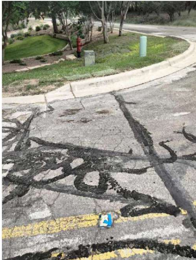
2024.05.16, Blue Reflector Marker at Lakeland Dr / Lakepoint Cir
