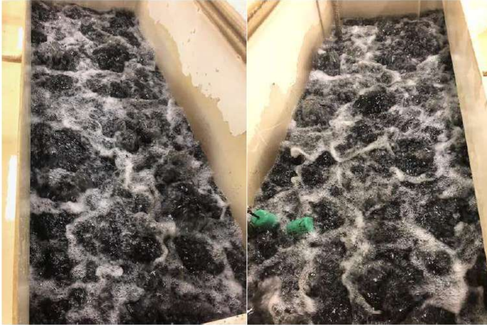
Filter during air scour
