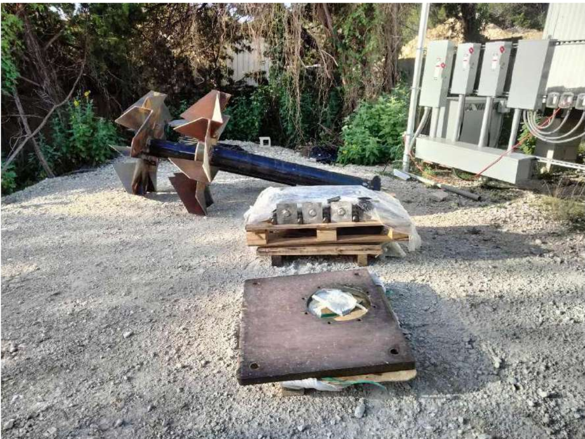
2024.07.01, Delivery of Mechanical Surface Aerators & Accessories
