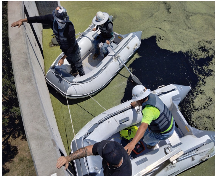
2024.07.18 - ACP Obtaining Field Elevation and Radial Measurements on Top of Wall inside Effluent Concrete GST
