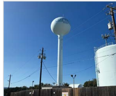
Comanche Trail Elevated Storage Tank
