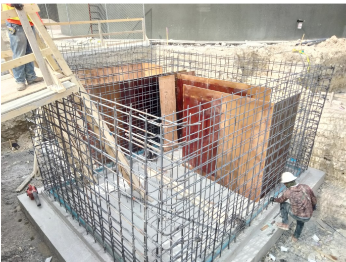
Chlorine contact/effluent transfer basin for new WWTP.
